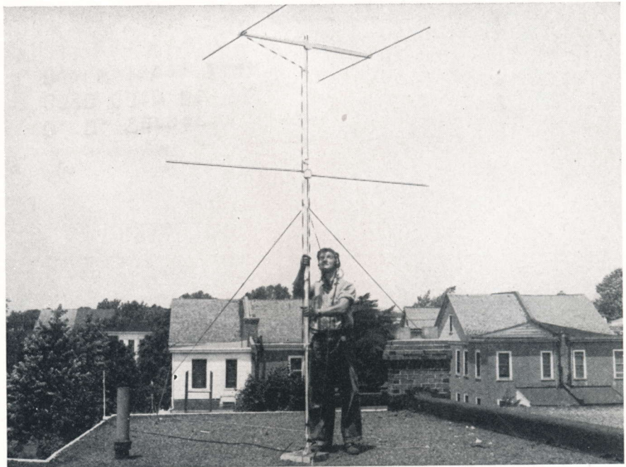
Philco aerial system being installed and oriented by a television serviceman. Two Philco aerials are mounted on the mast. At the top is a dipole with reflector, and at the center is a simple dipole.
