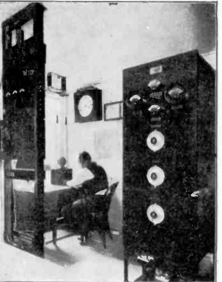
Fig. 3. Main control panels of a Radio Broadcast Station.
